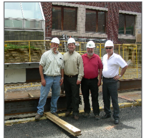
With Kendall Hotel owner, Nicholas Fandetti and Architect Gerry Fandetti, Sullivan team members sign and hoist the final piece of steel for the seven story addition.
